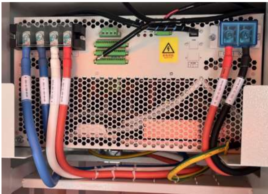
Figure 6.1: Completed wiring of the JKP-100LN-BA (back side view)
